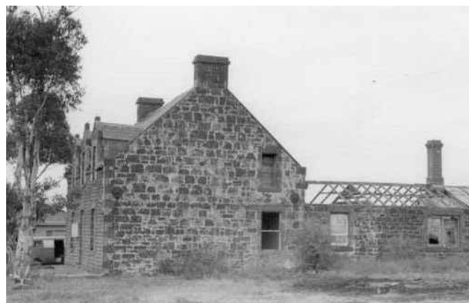
Figure 28: Gowrie, 63 Gowrie Street, Glenroy, prior to restoration, side elevation. Photograph by John Collins in c.1963. Source: J.T. Collins Collection, Pictures Collection, State Library of Victoria.
